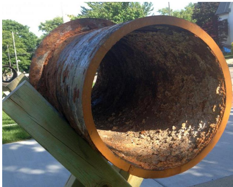
Figure 1.1 Increased roughness in pipe ([116])
