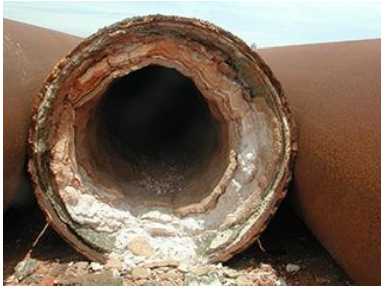
Figure 1.2 Partially blocked pipe ([40])
