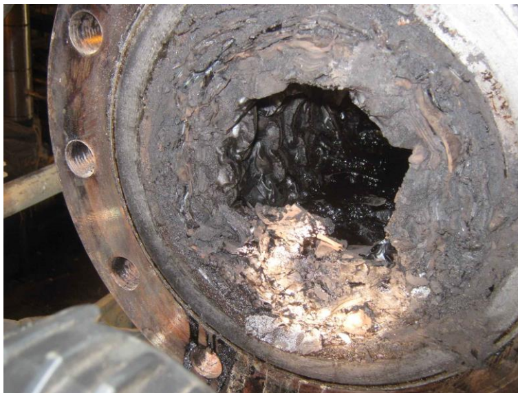
Figure 1.3 Severely blocked pipe ([128])
