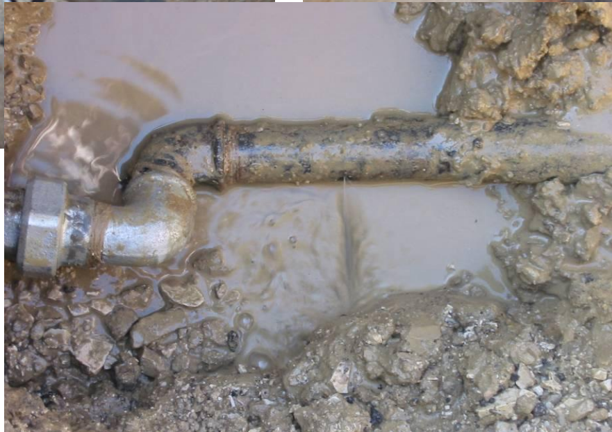
Small leak in the aqueduct of Perugia
